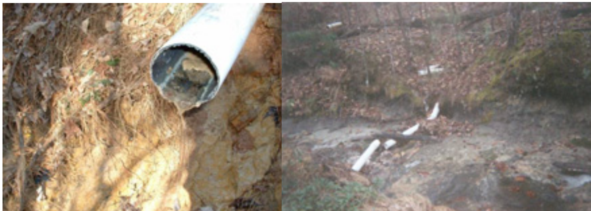
Figure 16: Failing sand filters (left) and sanitary sewers (right) pose health risks and harm water quality
