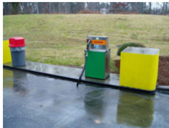
HS-3-5 Uncovered diesel fueling station at Hess gas station on U.S. 70
