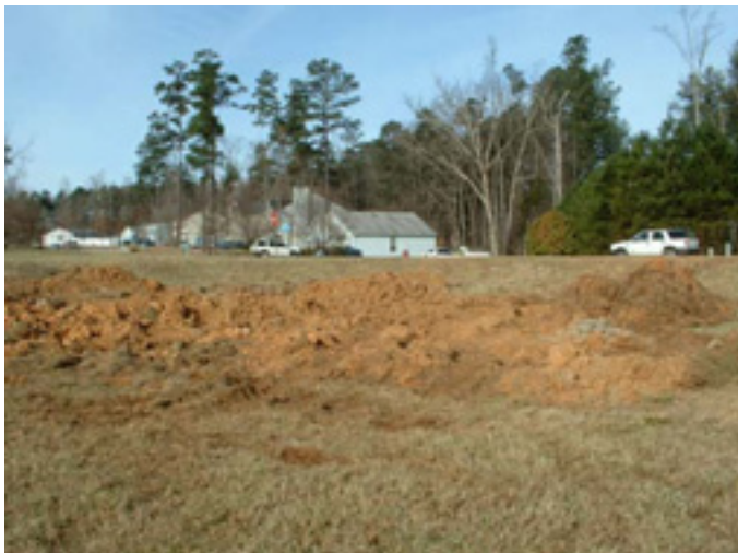
RCH13-1 No ESC provided for on lot construction (Photographer standing adjacent to stream channel)
