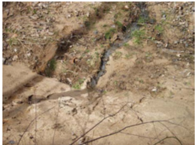
RCH3-2 Sanitary sewer leak: (UT3-1)
