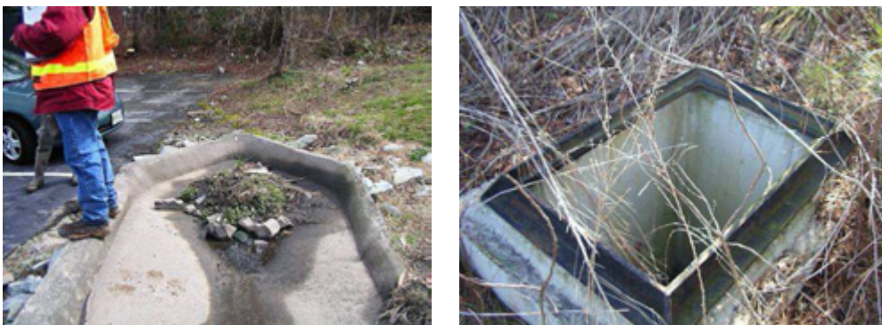
Repair projects include storm drain infrastructure such as this inlet at Pizza Hut (MI-306) (left) and stormwater management ponds (MI-320) (right).
