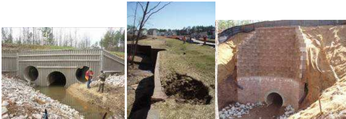
SC-301 Golden Parkway (misaligned culvert); SC-111 poor drainage design behind headwall of interlocking concrete block; SC-112 poor headwall design.
