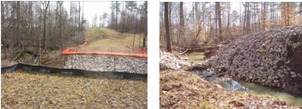
UT-303 (left) Sewer crossing in Brightleaf is one of three is close proximity. UT-110 (right) demonstrates the typical steep side slopes and small rip-rap.
